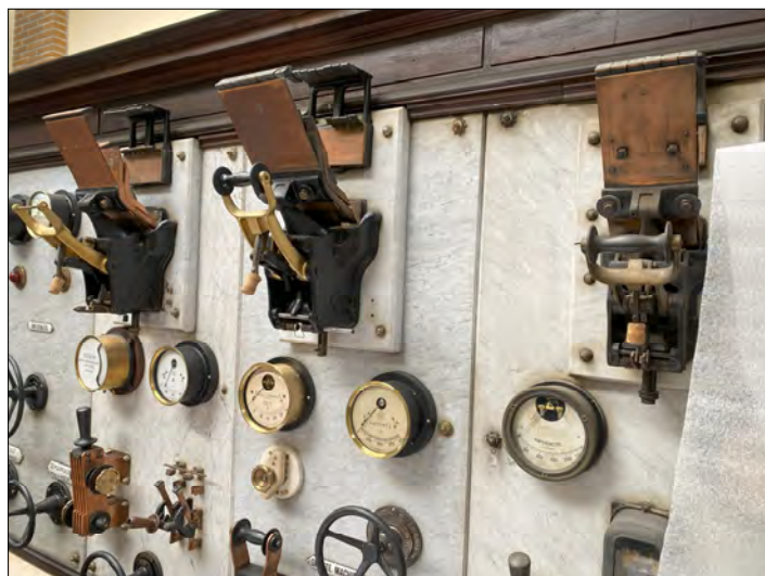
Part of the switch mechanism at the Izegem power station.
