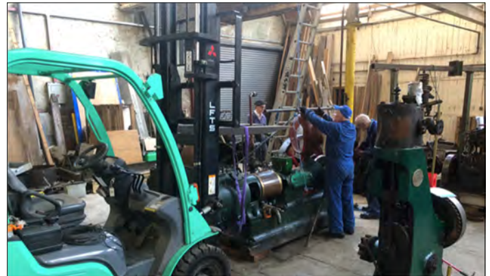
Restoration work underway on the shaft race roof. Image copyright Anthony Pilling.
