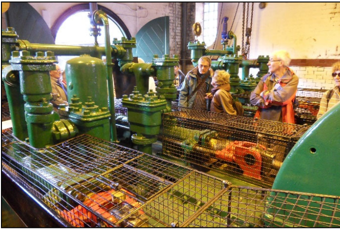
The New Pumps installed in 1907. Image copyright Ian Barclay.
