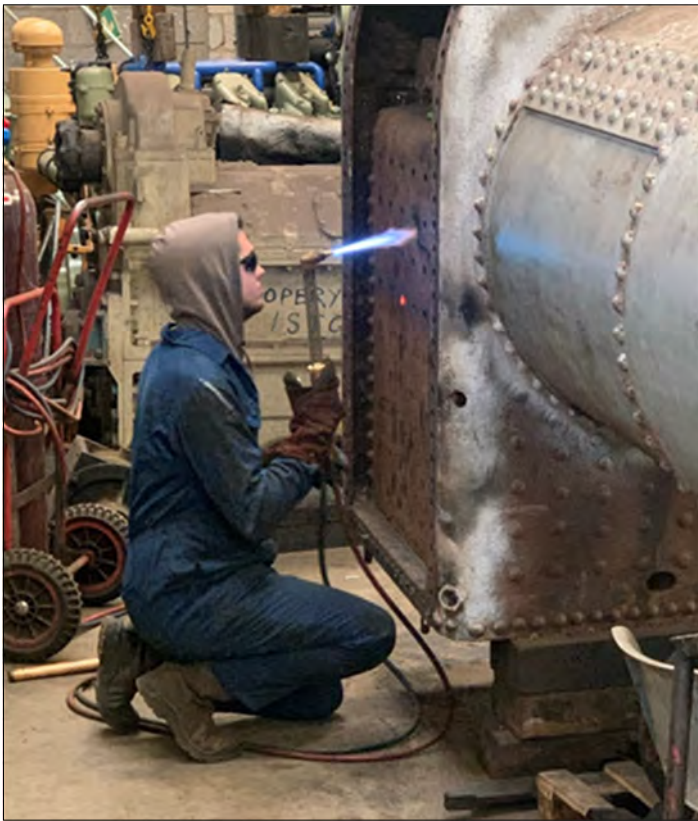
A volunteer working on repairing the boiler of the Hudswell Clarke locomotive.
