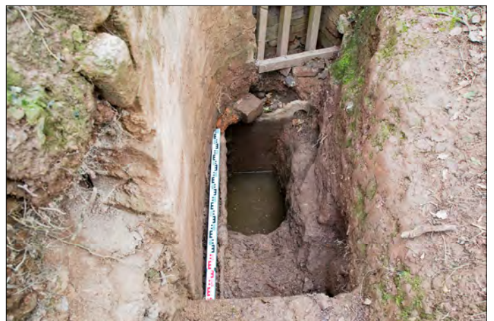
The condenser pit next to the pumping shaft.
