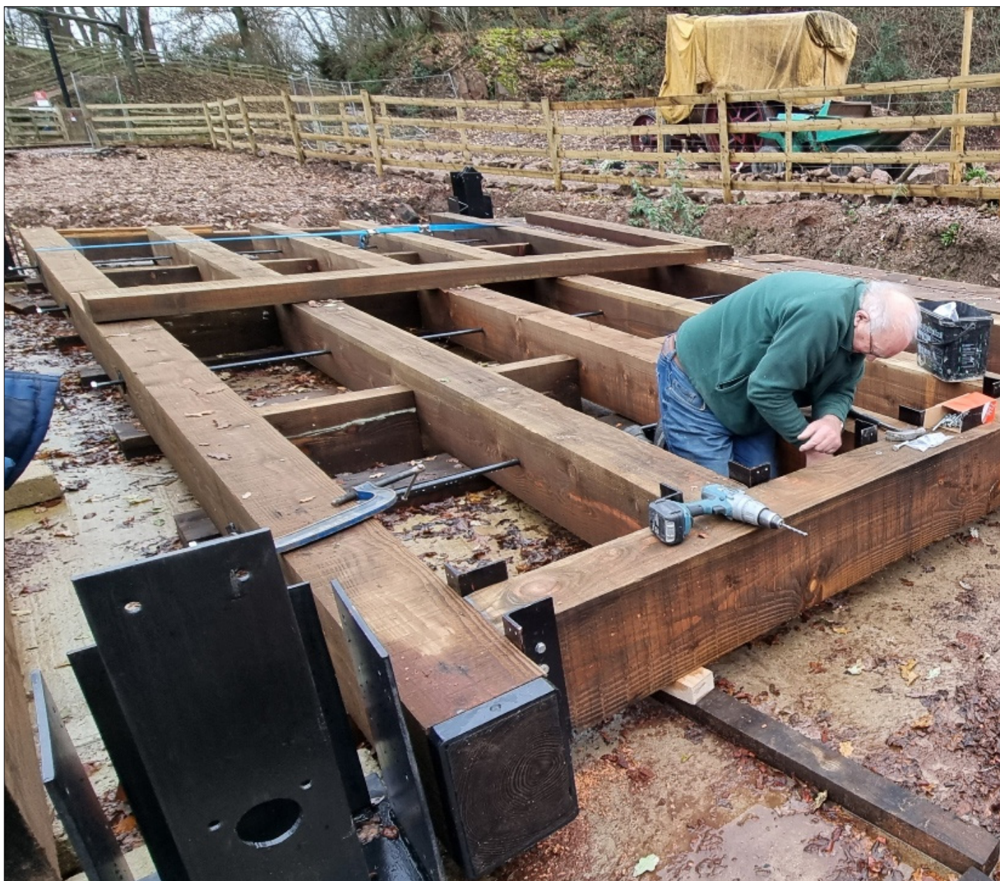
The new timbers being fitted to the iron framing of the Stevenson Lifting Bridge. Image Copyright Steve Cramp.
