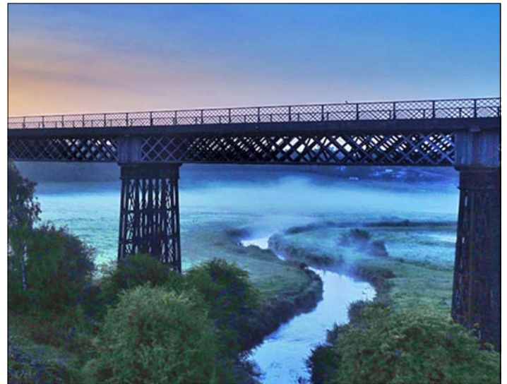
Bennerley viaduct in the mist (picture credit Paul Atherley, Friends of Bennerley Viaduct)
