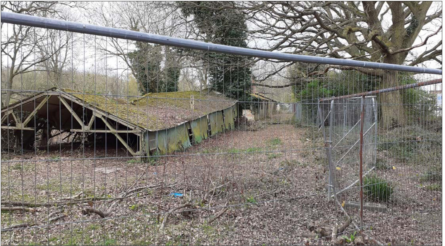
The Guard's compound showing the poor condition of some of the buildings. Image courtesy of Tony Crosby.
