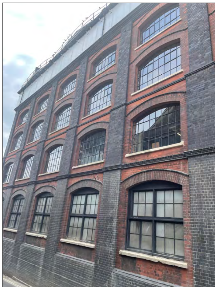
The restored northern elevation of the Pattern Store. Image courtesy of Diocese of Bristol.
