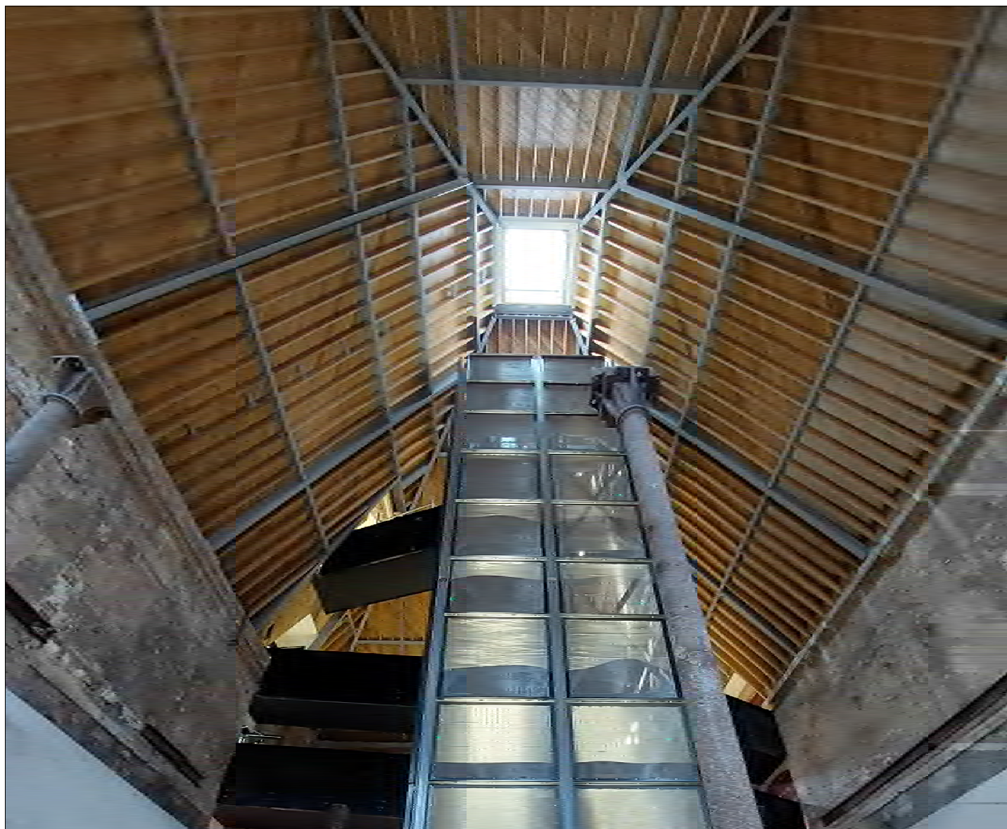
The interior of the kiln at Shrewsbury Flaxmill Maltings showing the roof structure and the newly inserted lift shaft.
