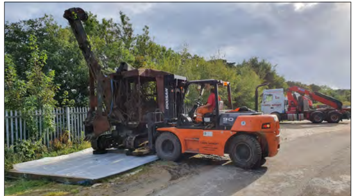
The tracked bucket excavator being moved to its concrete plinth. Copyright: NCMM.
