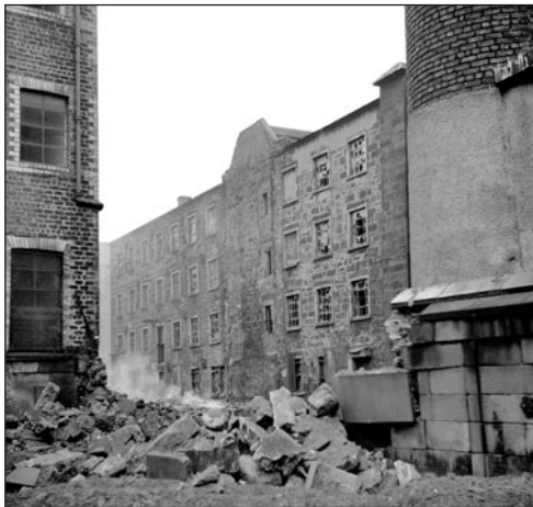
The former Bishop Garden Weaving Factory, Anderson, Glasgow, immediately prior to demolition, 1966
