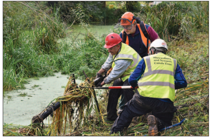
Shrewsbury & Newport Canal Society along with Waterways Recovery Group (WRG) and National Trust Archaeologists working on clearing the canal at Berwick Wharf, Shrewsbury Canal, Attingham, Shropshire. 12/10/2019
