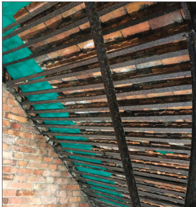
Roof tiles on unsecured laths
