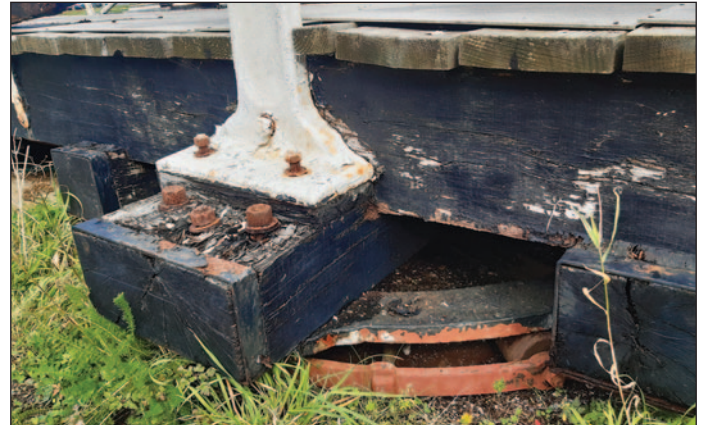
Timber decay to main pivot beam
