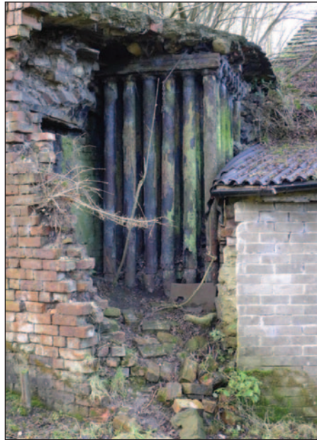
Remains of an economiser exposed at the base of the chimney at Dale End Mill, Lothersdale
