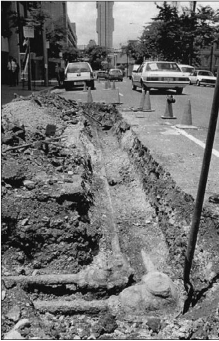
Part of the 1992 excavation – looking south-east along William Street from the corner of Stephens Lane. Note the shallow depth of the excavation below the road surface, and the right-angle joint 'boxes' for the 2-core and 3-core Tubes. Photo: Courtesy of EnergeX.
