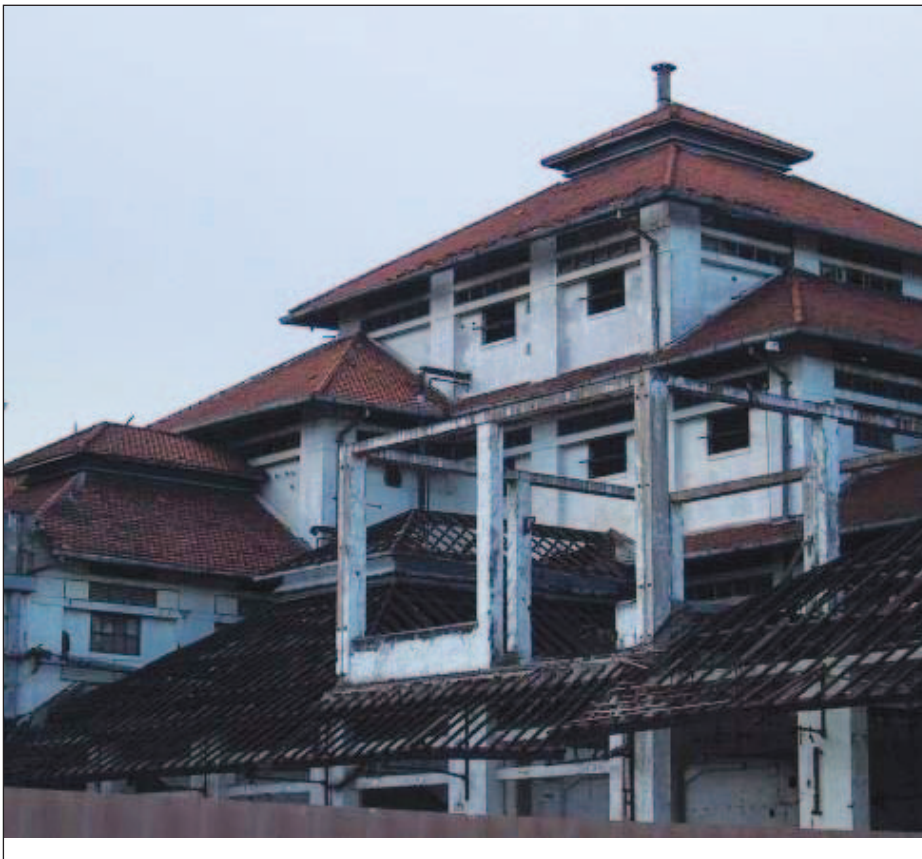
Brewery in Surabaya, East Java, Indonesia, during demolition after the factory was relocated in 1988 and the site was converted into commercial complex 2000 photo author
