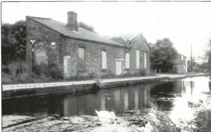
BO42: Bolton, Bury and Manchester Canal - stables, workshop and lock keepers cottage. Photo David Lewis
