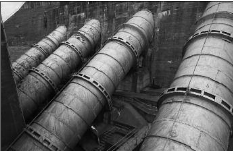
Penstocks at Ardnacrusha able to delivery 100 tons per second
