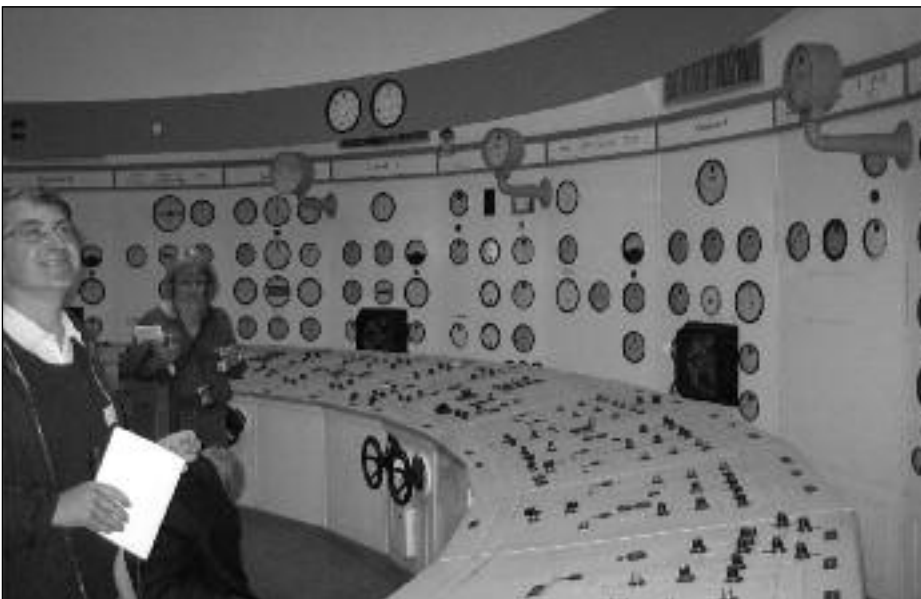
Original Control Room at Ardnacrusha Power Station
