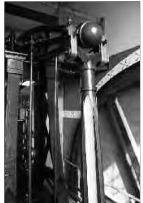
The beam engine at Dogdyke pumping station
