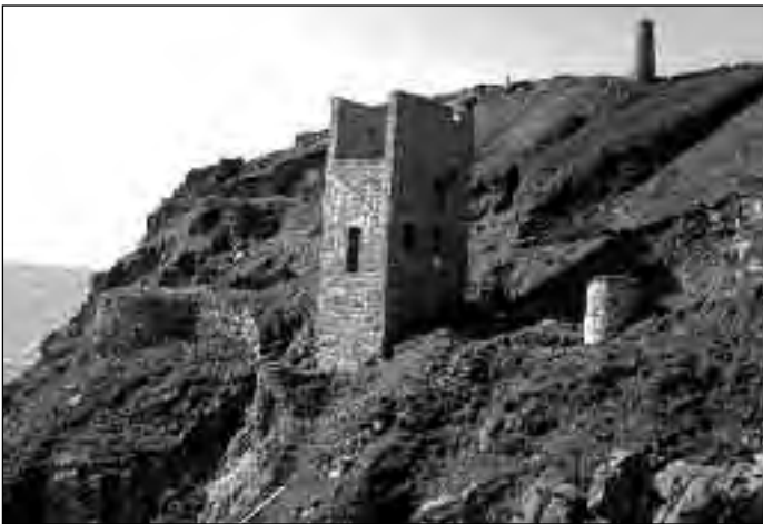
Conservation work has now been completed by the National Trust at the Old or West Engine House, the adjacent whim plat and stack at Trewavas Head Photo: Sid Geake
