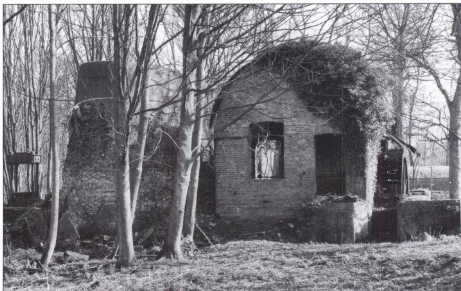
The Press House, Royal Gunpowder Factory, Waltham Abbey, Essex. Waltham Abbey was a model example of how detailed recording can inform co-ordinated statutory protection. The 71 hectare site contained over 300 structures and features and more than two thirds of it was designated a Scheduled Ancient Monument with 21 listed buildings. The gunpowder press house, which retains its waterwheel, hydraulic pumps and press, was built in the mid-1850s and is the sole standing example of its type in England.
