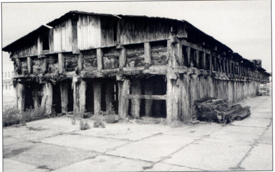
Concentrated brine from the gradation towers is held in wooden holding tanks before passing to the saltworks Photo: P. Graham
