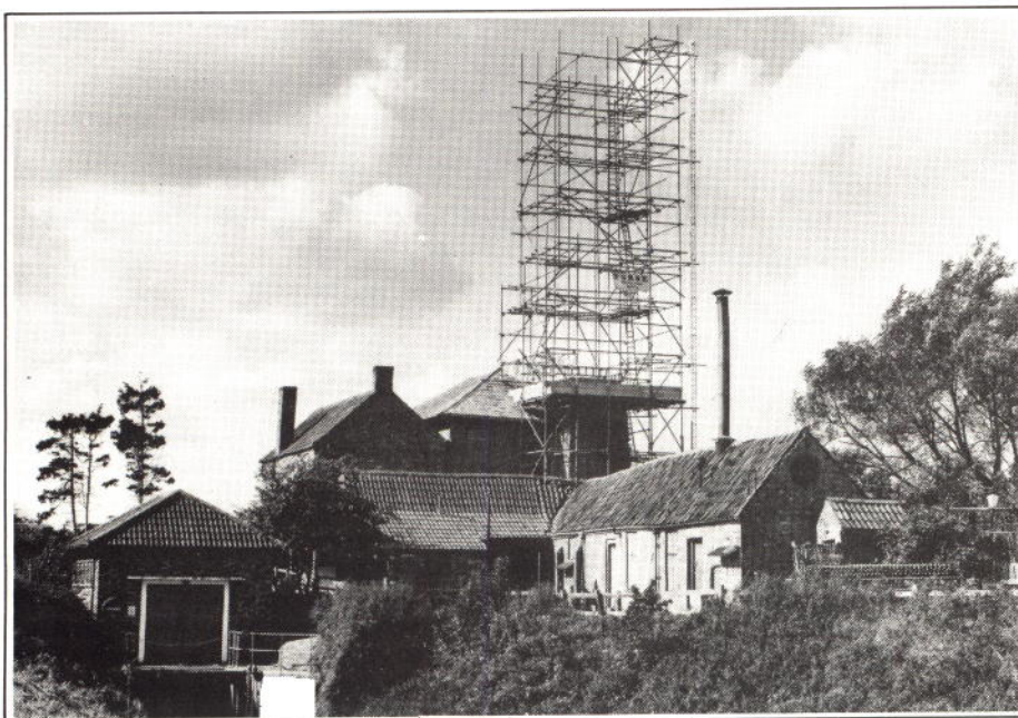
Hole in the sky: the main stack at Westonzoyland after dismantling and shortly before re-erection. Photo: Ian Watts
