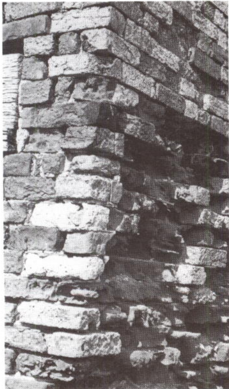
Dauntsey Lock, Wiltshire: Erosion of salt-store wall.
