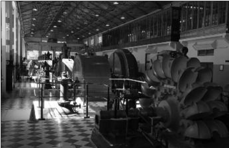
Waddamana 'A' Generator Hall with Pelton wheel
