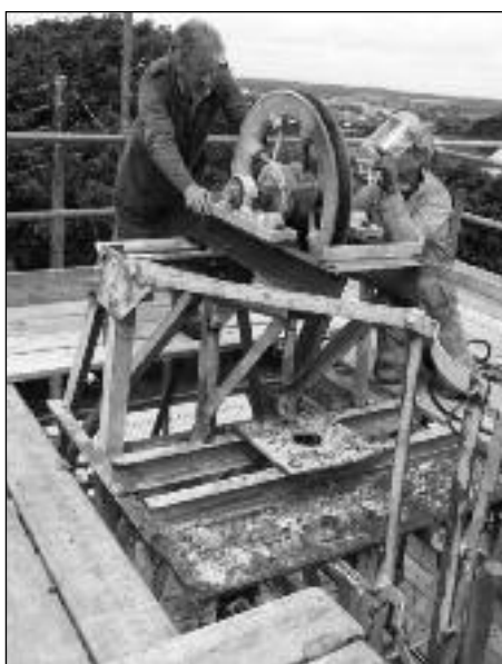
Great Condurrow Mine, 4th August 2011. Huw Rowe and Bob le Marchant inspecting the sheave wheel on top of the headframe after it had been scaffolded
