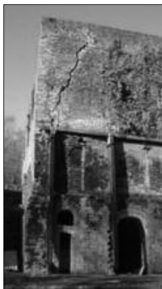
Amberley – De Witt lime kiln. The damaged SE corner before repair Amberley Museum and Heritage Centre
