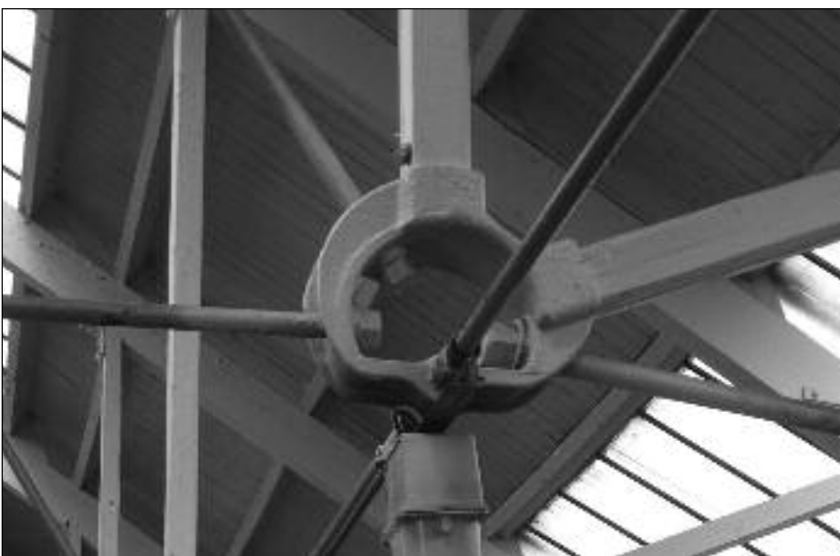
Old Oak Common, early and unusual cast steel nodes connecting steel tie-rods and timber struts in the roof trusses of the Stores building
