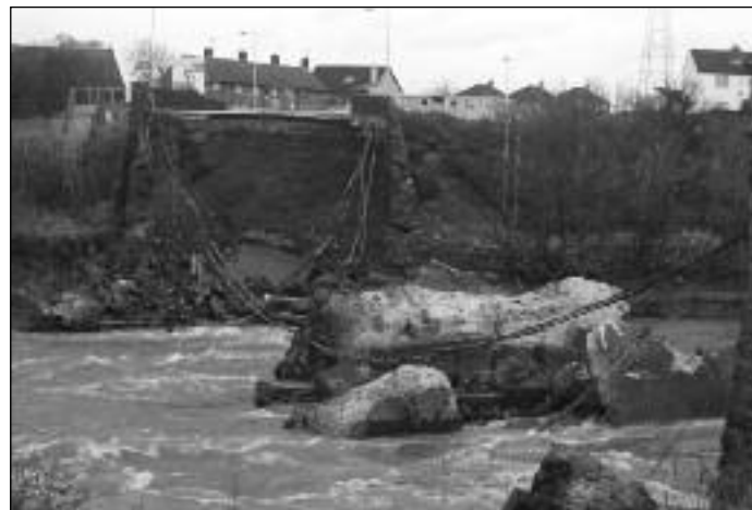
North Bridge Workington, destroyed by floodwater
