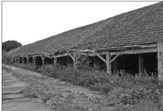
The condition of the former rope walk at the Parrett Works is a cause for concern Photo: Geoff Fitton
