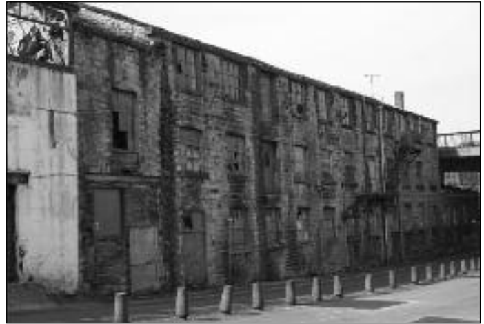
The early mill building, possibly a hand-loom weavers shop, in Exmouth Street, Burnley, which has been demolished over the past year Photo: Roger Holden
