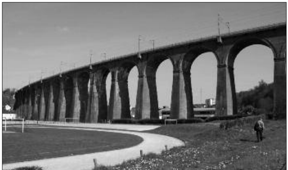
The great Barentin Viaduct, designed by Joseph Locke and originally built by Thomas Brassey in 1846. It was rebuilt after an early collapse Photo: © Bill Barksfield 2010
