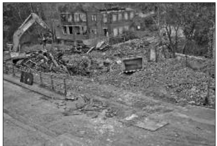
The appropriately named Complete Demolition contractors completing the demolition of Middle Mill, Hopes Carr, Stockport, after the fire of 26 November 2009. Note the burnt-out shell of another building behind, the result of an earlier fire
