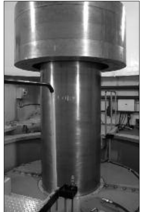
Shaft and upper housing of a turbine in Ohau B power station Photo: Fred Barker
