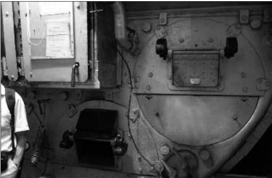
The two right hand boilers of the Lyttelton tug, the higher one being a challenge to the stoker
