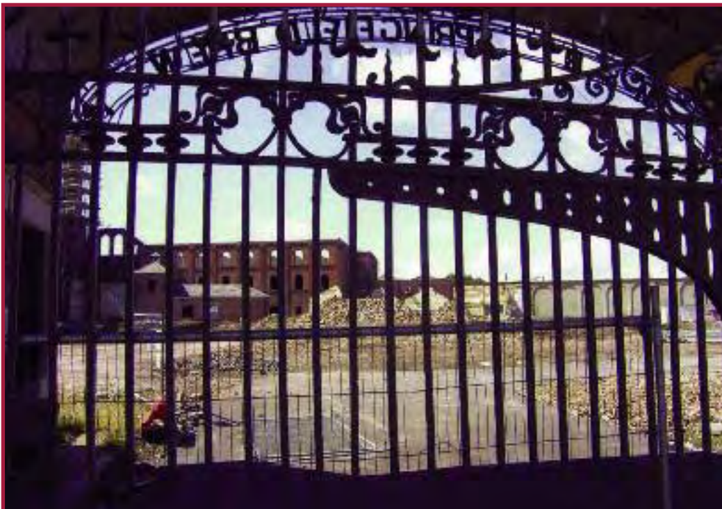
Demolition at the gates: an increasingly common scenario? Fortunately, Wolverhampton's Springfield Brewery was recorded on film in better days (see inside, page 12)
