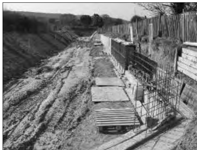
Restoration work in hand near Drayton Beauchamp on the Wendover Arm of the Grand Union Canal Photo: Henry Gunston
