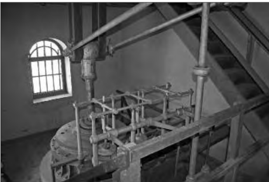
The Harvey 50-inch engine inside its house at Okiep. It is claimed to be the only Cornish engine surviving in situ in the southern hemisphere
