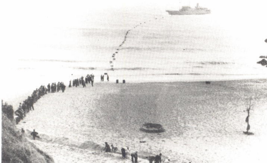
The Cornish seaside: bringing a submarine cable ashore at Porthcurno beach, c1952
