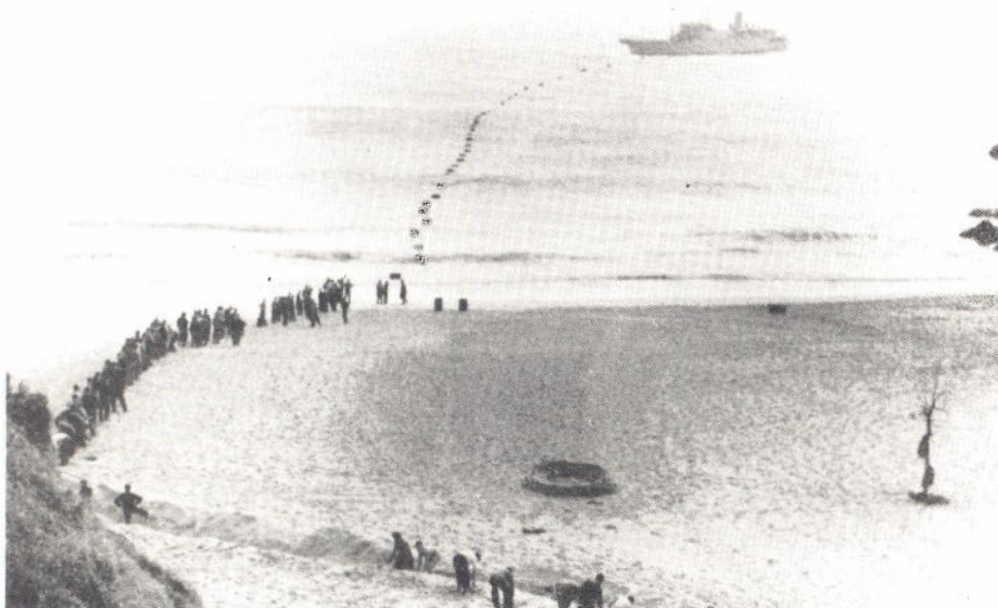
The Cornish seaside: bringing a submarine cable ashore at Porthcurno beach, c1952 Photo: The Trevithick Trust
