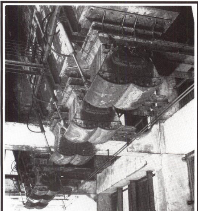
Colliery recording in Wales, October 1992: an underside view of hydraulically operated doors of the rapid rail loading bunkers at Taff Merthyr Colliery, Mid Glamorgan, which closed last year and is under demolition. There are three glass-lined bunkers, with a combined capacity of 2,000 tonnes of coal, and each 28-wagon train was loaded and weighed while on the move. Aberthaw Power Station near Barry took the entire output from the colliery at the rate of one 900 tonne train each day. This photograph is part of the survey of Taff Merthyr Colliery carried out by the Royal Commission on the Ancient and Historical Monuments of Wales, is in preparation for the Commission's forthcoming publications on collieries. The first of these is due for distribution through Alan Sutton Publishing later this year, Colliery Architecture and Engineering in Wales.
