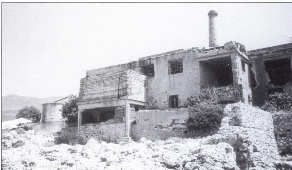
Kardamyli Soap Factory viewed from the west. The first phase soap preparation building is in the centre, with adjoining reinforced concrete oil fuel tank and pump house. The second phase extension (right) displays possible war damage
