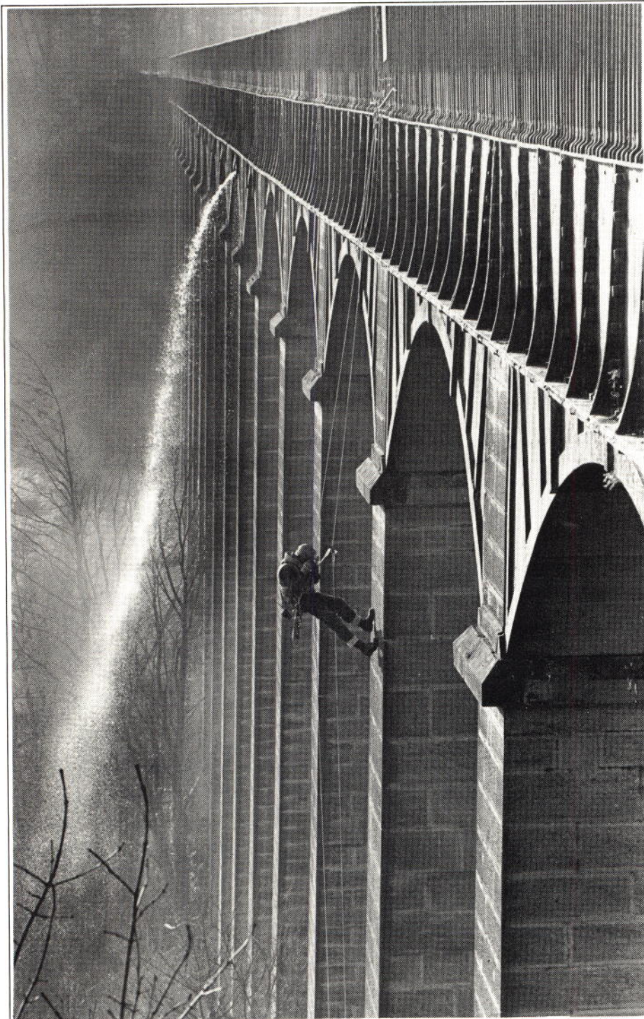
Engineers do it Abseiling, a civil engineer inspecting the pillars of the Pontcysyllte Aqueduct on the Llangollen Canal. Photo: courtesy of Waterways News Copyright BWB.
